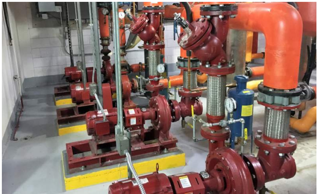
HYDRONIC PUMPS at OSBORN 360 // St. Paul, Minn.
