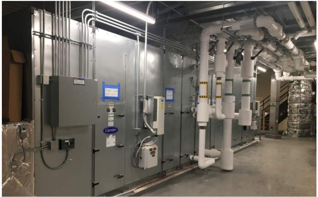
AIR HANDLING UNIT AND HYDRONIC PIPING at SMSC // Shakopee, Minn.
