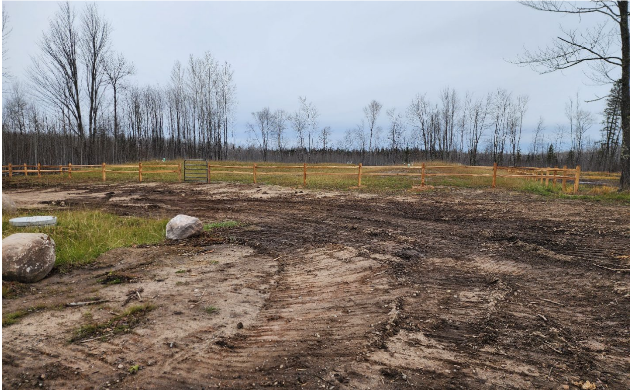
Photo 4: Fencing at New Septic Mound System for Campground ISTS/SSTS
